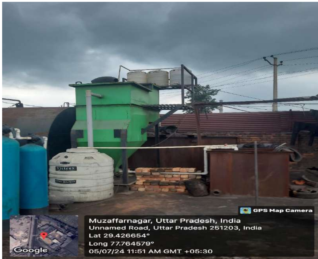
Figure 7 Installed ETP under trial
