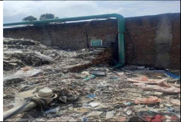
Borewell-2 defunct flow meter
