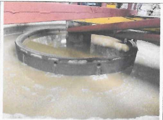
Photo 6: Overflow tank cum storage for recycling
