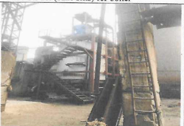
Photo 10: Gasifier for plastic waste
