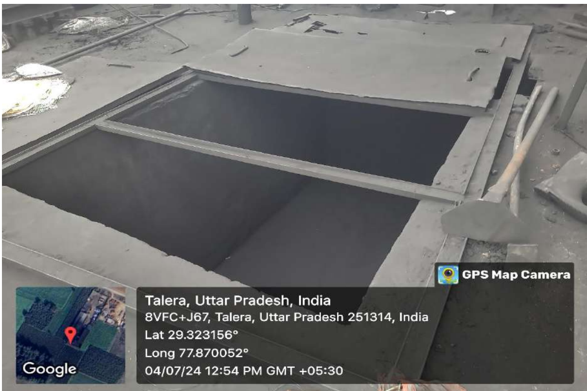
Figure 8 Char storage tank
