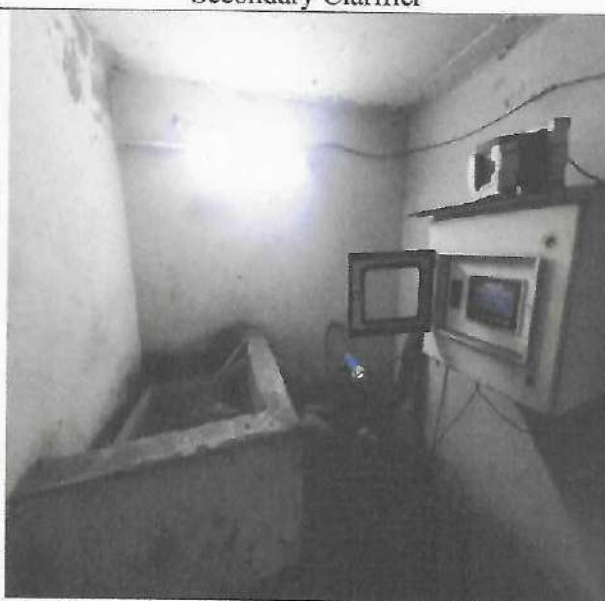
Flowmeter and OCEMS at ETP outlet
