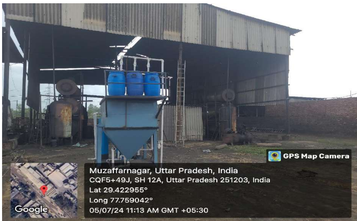
Figure 6 ETP under commissioning
