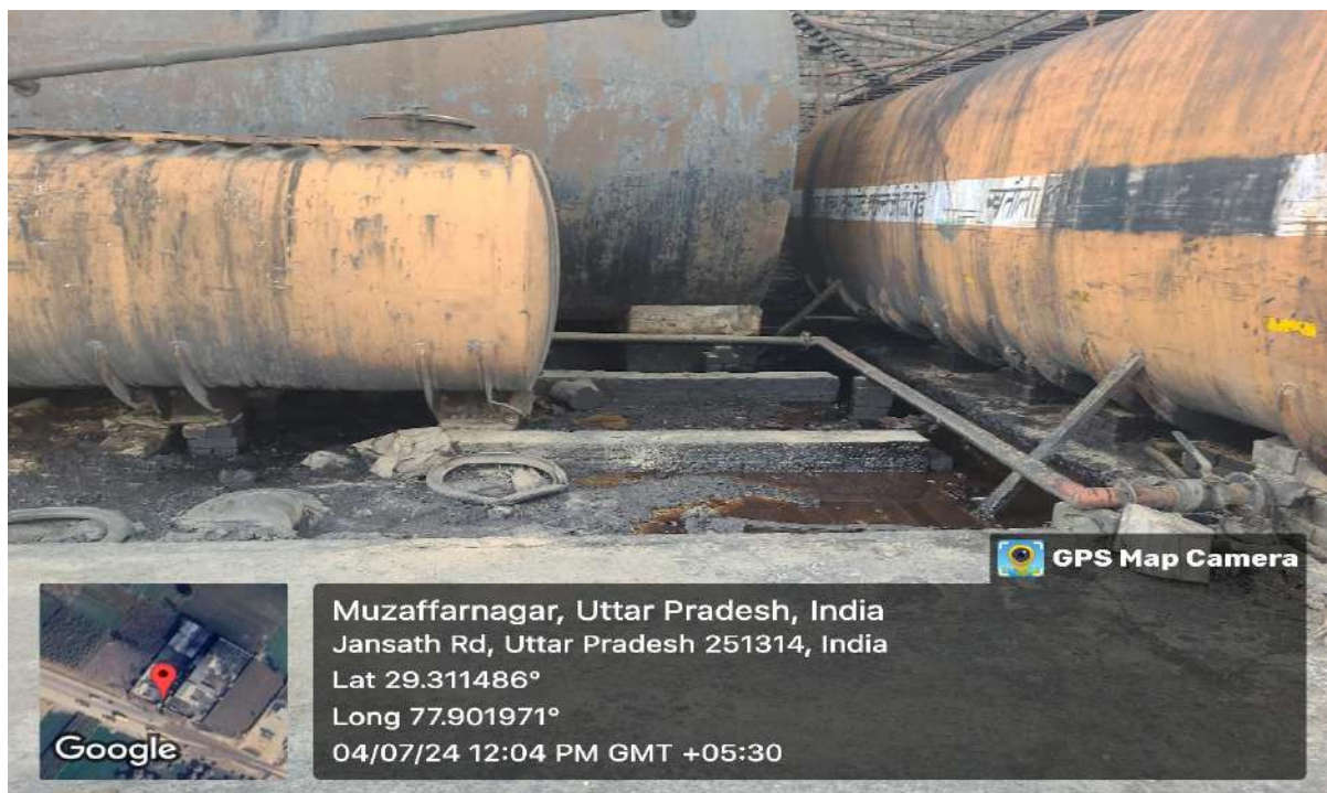
Figure 2 Empty oil tank inside unit premises
