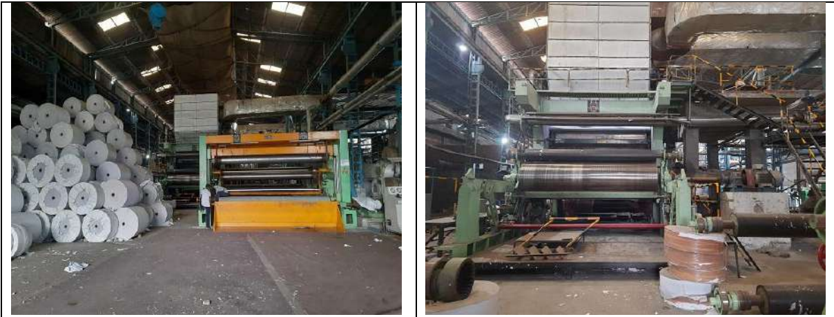
Non-operational machinery at unit
