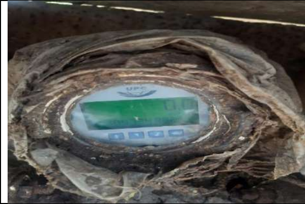
Flow meter installed at Borewell-1
