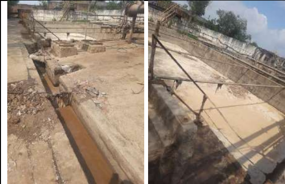
ETP Inlet & Equalization tank
