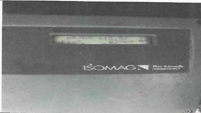
Photo 7: Flowmeter at recycling line after sedicell
