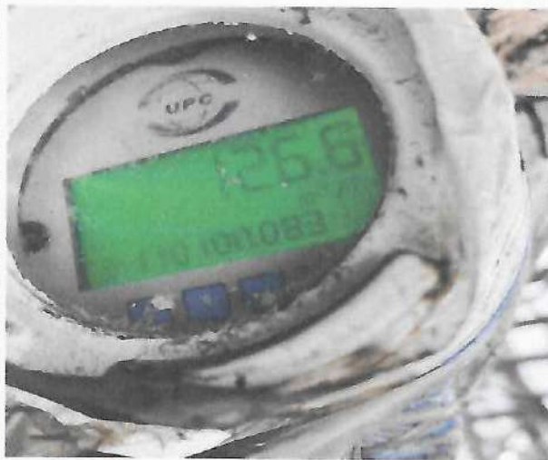
Flowmeter reading of ETP inlet
