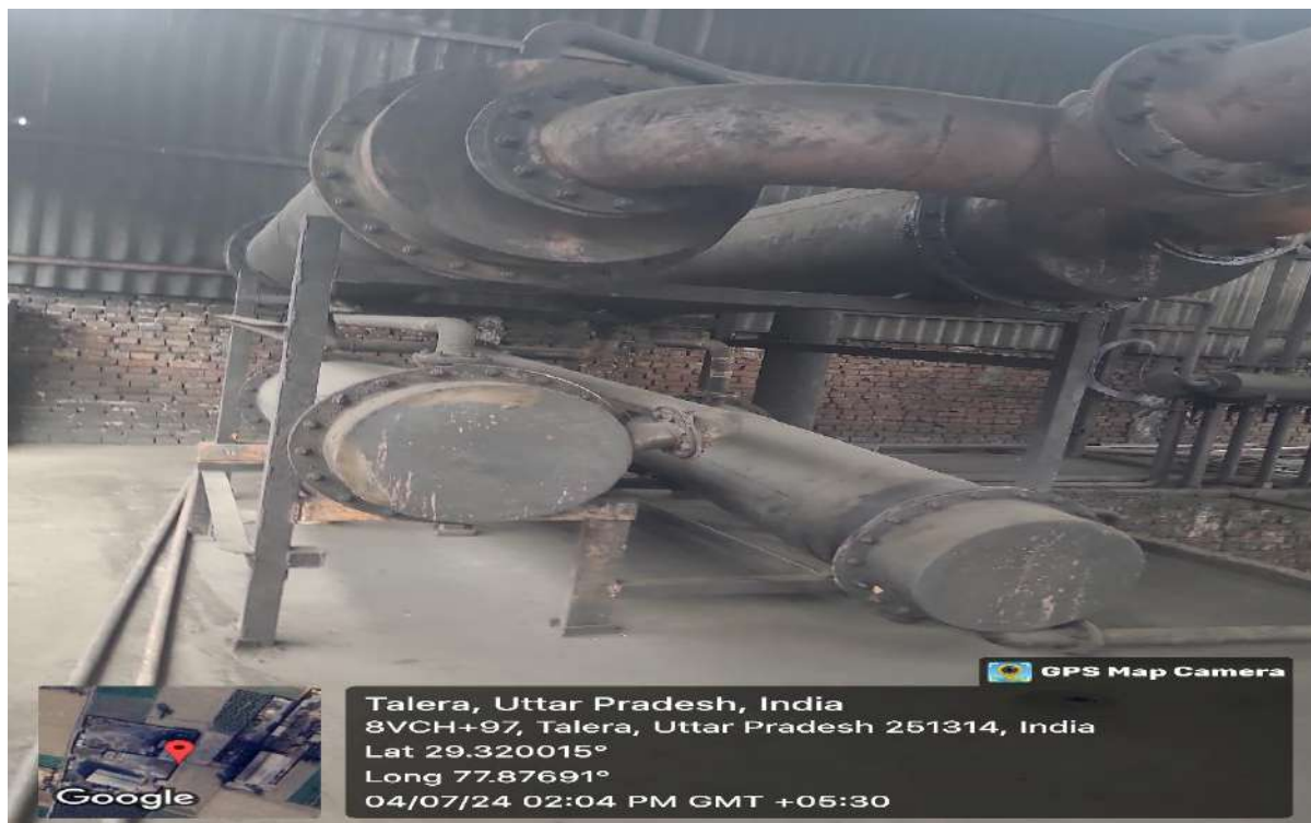
Figure 8 Oil and gas compressor system
