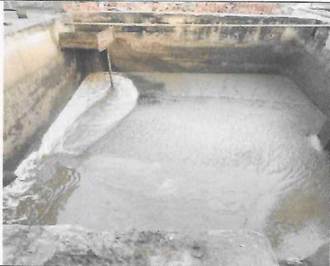
Photo 3: ETP inlet channel
